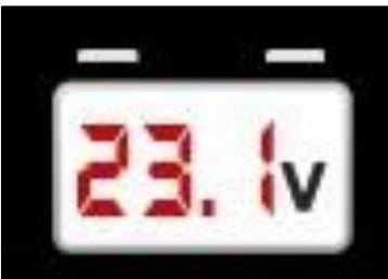
[Fig. 3-23] Battery Voltage
